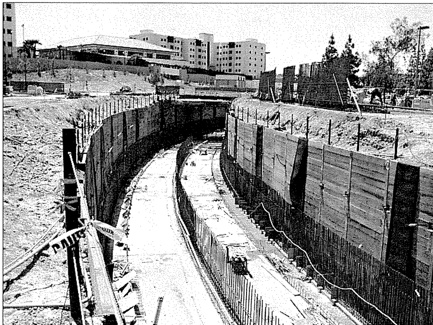
Cut and cover portion of the SDSU tunnel alignment. Photo by Robert Stroh.
