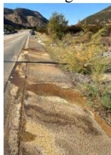
Fig. 1. Seeps along Old Highway 80.
