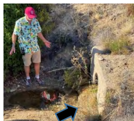
Fig. 2. Culvert filling with calcareous tufa.
